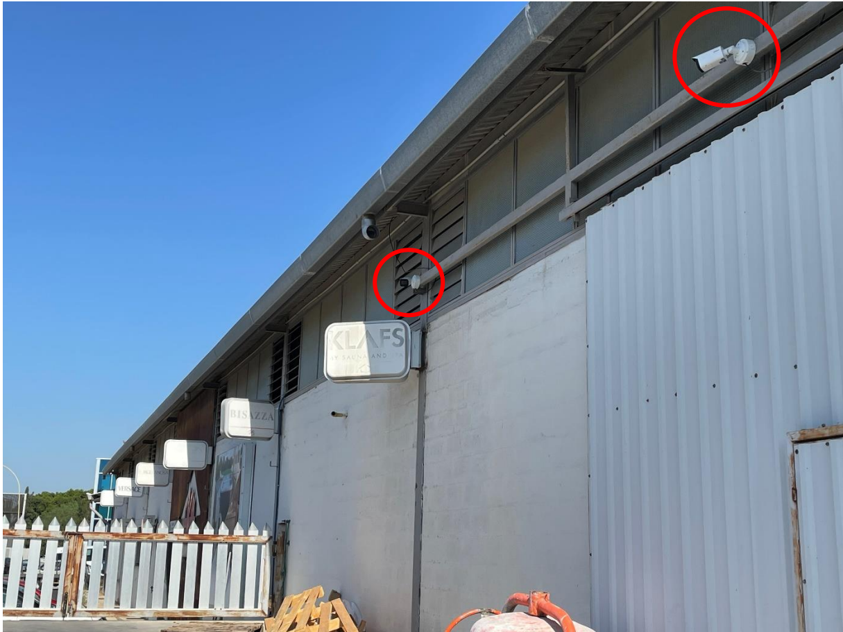
Figure 6 DAHUA Network Cameras, outdoors, facing entrances and corridors
