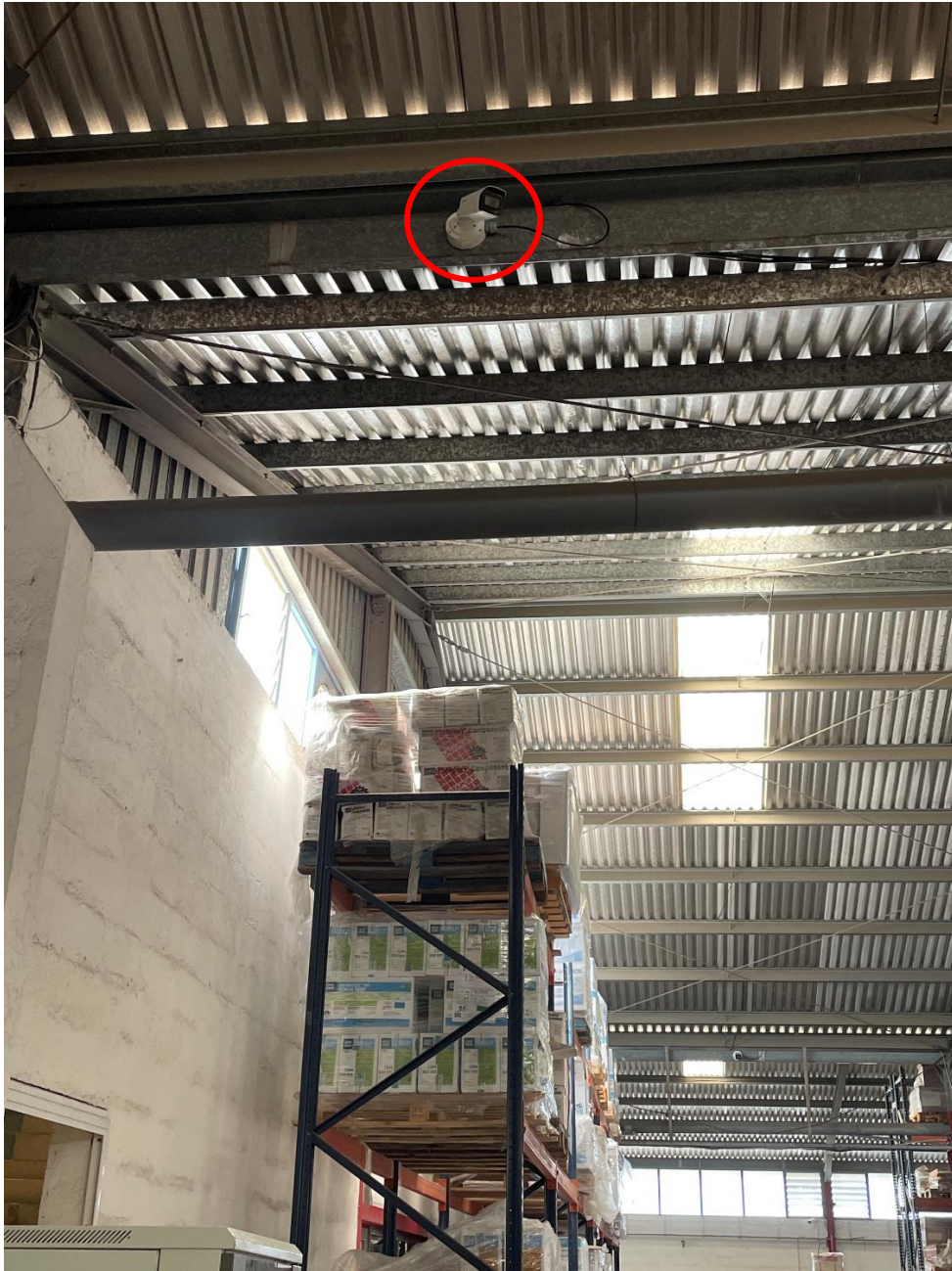
Figure 5 DAHUA Network Camera, indoors, facing entrances, shelves, and corridors
